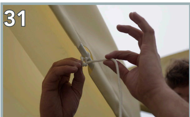
31 Using the Long Rope on the front of the pergola, tie it to the Pole that is in front of it. Repeat this process for the Small Rope to the Pole cutout futher along.
