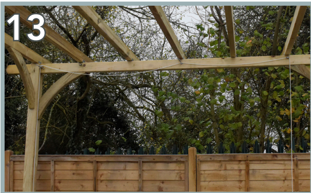
Repeat the process for the front and back of the Pergola. Ensure it looks like the above.
