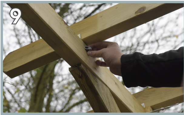
Position 1 x Small Roller centrally under the first rafter inwards from each upright post. Secure using 2 x 35mm screws each.
