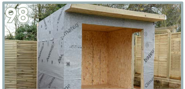
The final result is shown above. You do not need to add membrane to the canopy / the roof overhang.
