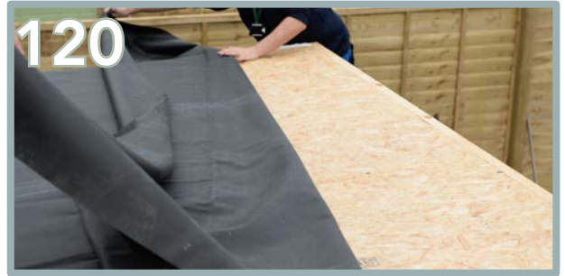
Fold the EPDM back to half way across the roof - we recommend two people for this. Be careful when moving on and around the roof to prevent any possible injuries.
