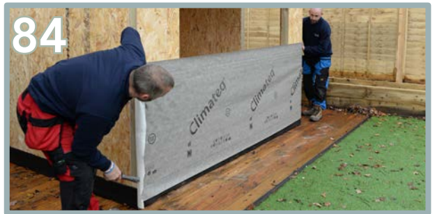
84 Starting with the bottom section, pull the membrane tightly and staple into place.
