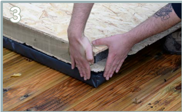
3 Ensure the panel is flush around the edges to the first bearer. Ensure the floor panels on the bearers are level using a spirit level as a guide.
