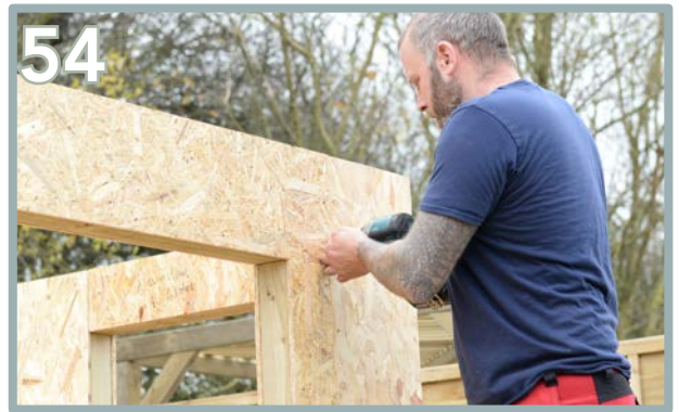
Position the screws on the Lintels OSB and screw into the wall batten behind. Secure into place using 4 x 35mm screws internally and externally, 2 x 35mm screws each side of the lintel insert.
