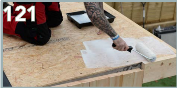
Pour the glue into a paint tray and use a roller for easier application.
