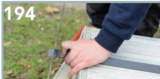
194 The side plastic trims for the door and window sizes will need to be trimmed down further to fit. Mark out your required length and cut.
