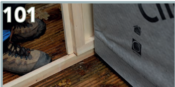
Repeat the same process for the second back panel (BI). Softly knock the second back panel into the first, so the T&G interlocks the panels together. Use a rubber mallet for a softer application. Repeat the same process for the (AX) T&G panel.
