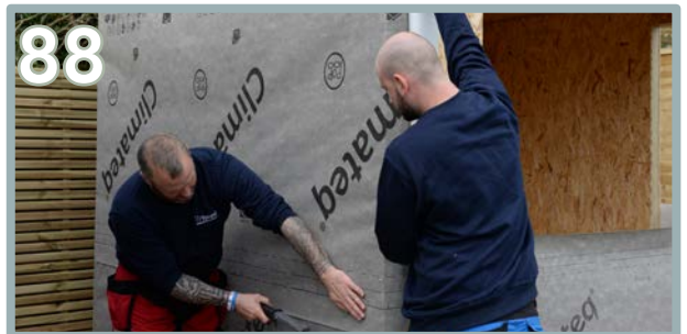
88 Repeat the same process for the top half of the building. Ensure the starting point is flush to the top of the back wall panels.
