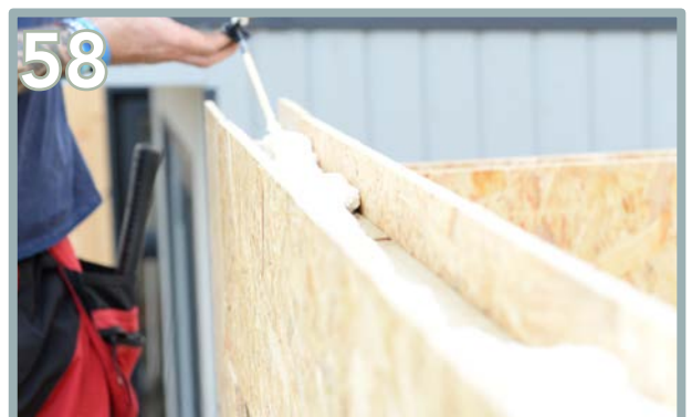
Use the expanding foam into the top groove, ready for the wall plates. Start at the front.
