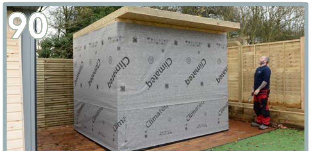
90 There will be a slight gap at the front and on the sides due to the angle of the roof.
