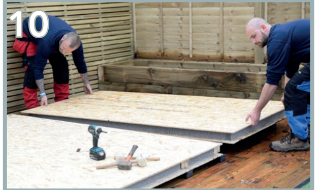
Place the fourth floor panel (F), knock into the second panel and ensure it sits flush on the final floor bearer. Repeat the process using 35mm screws in between the second and third panels.
