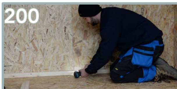
200 Repeat the process with the batten being flush to the bottom and end to end. Use 5 x 80mm screws along the batten at equal spaces.
