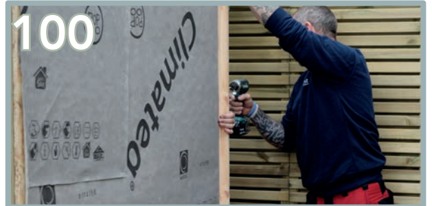
At each side, there will be a slight overhang of the T&G board. The battens edge underneath should be flush to the end. Use the 45 x 28mm batten as a guide to leave 45mm from the ground.
