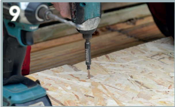
Using 4 x 35mm screws, pre-drill and screw where the adjoining panels intersect. This will secure the floor panels together. Repeat the same process for the third panel (E).
