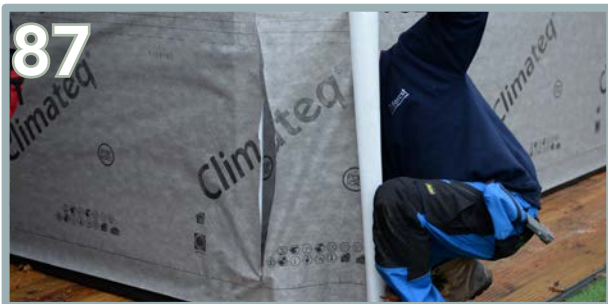
87 Once the starting point has been overlapped, cut off the excess and staple the end of the material into place.
