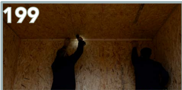
199 Begin at the back and position the 45 x 28mm batten flush to the top. This will be the correct length to fit in the space end to end. Use 5 x 80mm screws along the batten.
