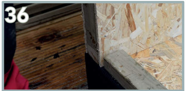
In the left hand corner, the wall panel will be flush to the edge and the floor plate as shown above.
