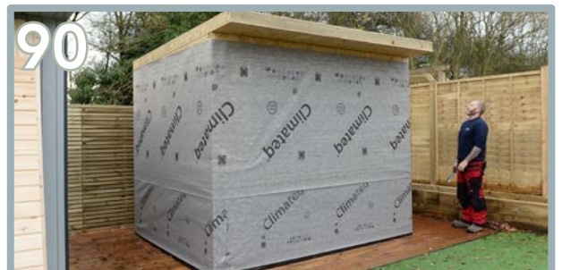
90 There will be a slight gap at the front and on the sides due to the angle of the roof.
