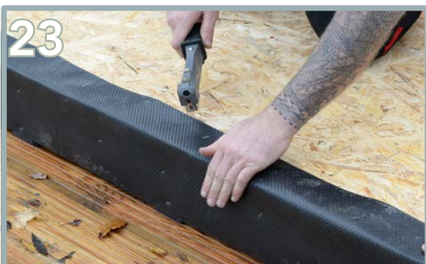
23 Continue folding the overhang and corners of DPC onto the OSB sheets as you make your way around and staple in place.
