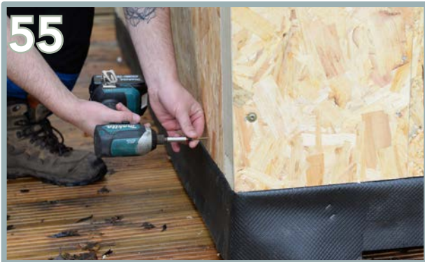
55 Once all of the wall panels are up, begin to secure each wall panel to the floor plate underneath. Use 3 x 35mm per panel externally.
