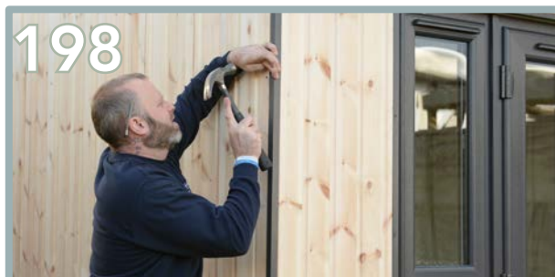
198 Add strips to each of the corners. The two on the back corners will be shorter. Trim to length if necessary and use 4 x pins.
