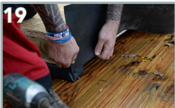
19 Start to unwrap the DPC roll and choose a starting point on the base's outer face. Ensure it covers half of the bearers and staple into place.
