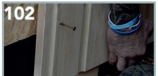
Use 6 x 80mm screws on each panel, 3 x 80mm down each side of the cladded panel, through the batten and into the wall panel behind. Leave the screws slightly out in case of adjustment.
