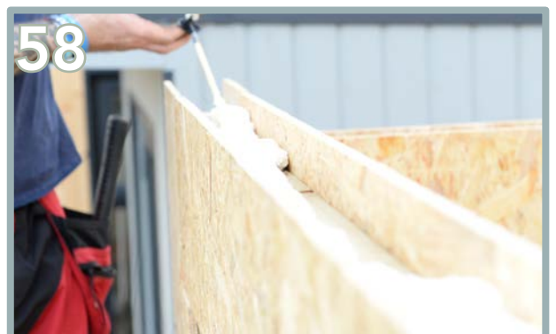
58 Use the expanding foam into the top groove, ready for the wall plates. Start at the front.
