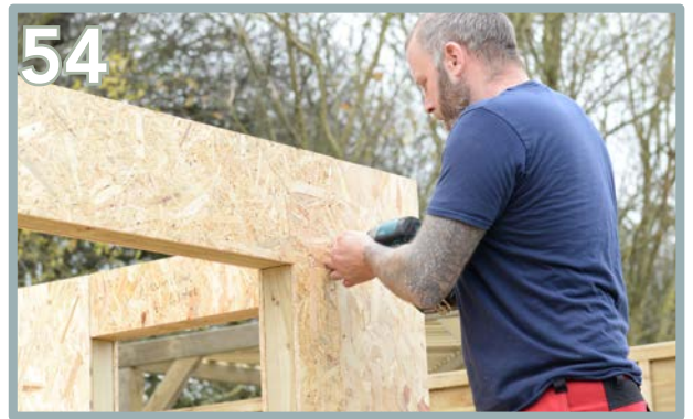
54 Position the screws on the Lintels OSB and screw into the wall batten behind. Secure into place using 4 x 35mm screws internally and externally, 2 x 35mm screws each side of the lintel insert.
