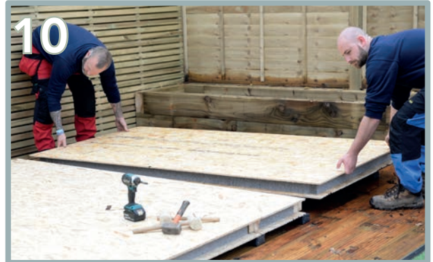
Place the third floor panel (B), knock into the second panel and ensure it sits flush on the final floor bearer. Repeat the process using 35mm screws in between the second and third panels.
