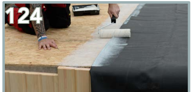
Repeat on the opposite half. Fold the EPDM back up until the point where the glue ended on the previous application.
