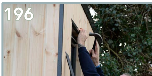
196 The same process applies for the window frame. Pre-drill and use 2 x pins on the front edge and 3 x pins underneath.
