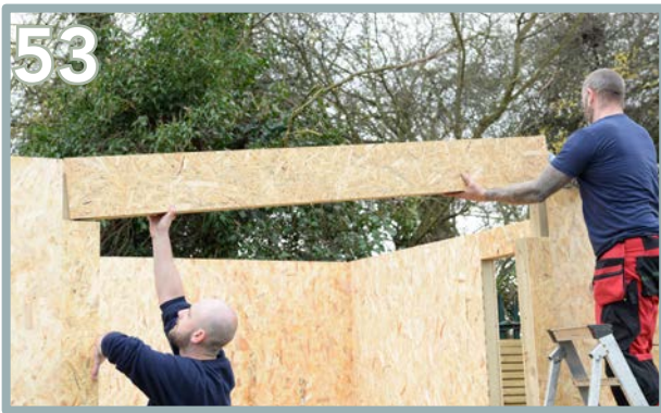
53 Insert the lintel piece (S) and knock into place. Ensure it is flush on the top.
