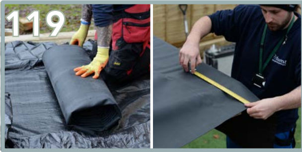
Unwrap the EPDM out onto the floor first, then measure out on the roof to ensure an equal overhang around all edges.
