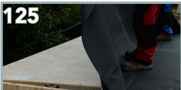
Continue with the glue application on the OSB roof surface as much as possible.
