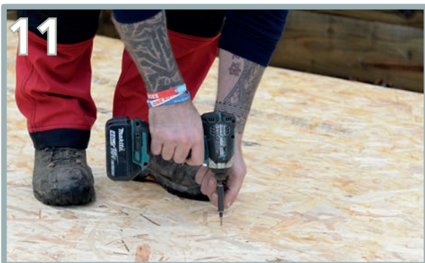
Once happy that all panels are in the correct positions, further secure with 5 x 125mm screws along the third panel edges and the first panels outer edge into the bearers beneath.
