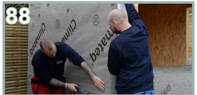
88 Repeat the same process for the top half of the building. Ensure the starting point is flush to the top of the back wall panels.
