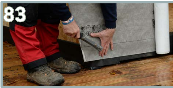
83 Begin to unwrap the breathable membrane. Position the membrane 45mm from the ground.
