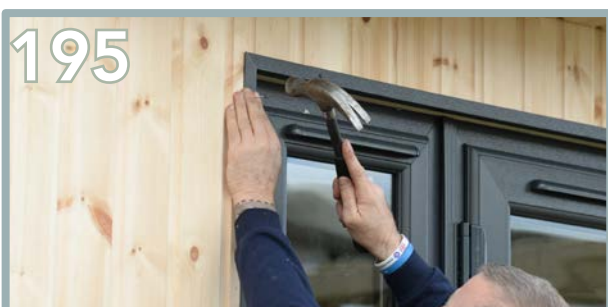
195 Use 5 x pins on the front down the side strip. Repeat the same process for the opposite side.
